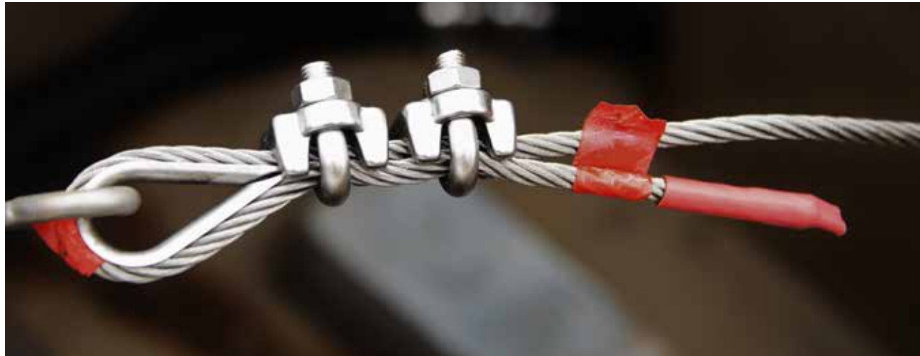
(5) The "dead end" of the cable has been marked with red tape. The wire clamps consist of a U-bolt and a saddle. These clamps have been installed properly, with the U-bolts on the dead end of the cable and the saddles on the working or standing side of the cable.
