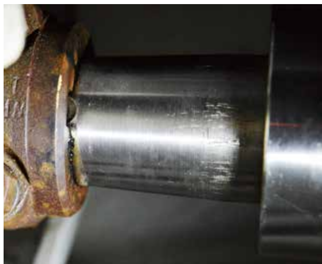
(7) A pipe wrench has badly scarred this shaft. In the area of the shaft seal, such scars can cause leaks and excessive wear on the seal. Shaft scars on the underwater portion of the shaft can lead to corrosion and micro-fractures, resulting in a broken shaft.
