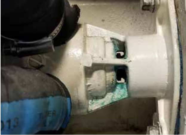
The engine seawater pump has openings which will reveal oil or seawater leaks through failing seals. The green verdigris in this image points to the seal on the seawater side.
