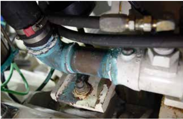
You don't have to see water to know there is a leak. Weeping connections at this oil cooler have taken a toll on the engine mount below it.
